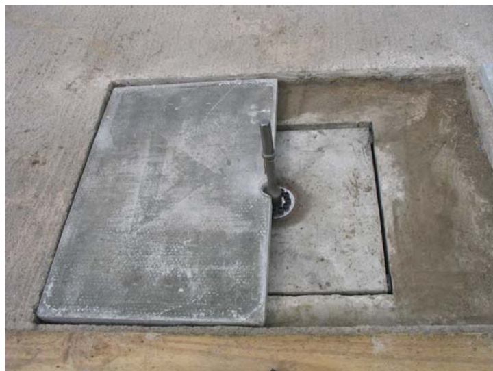
Figure 3a: Screening slab constructed in two halves – one half fitted over concrete block to show construction and placement
