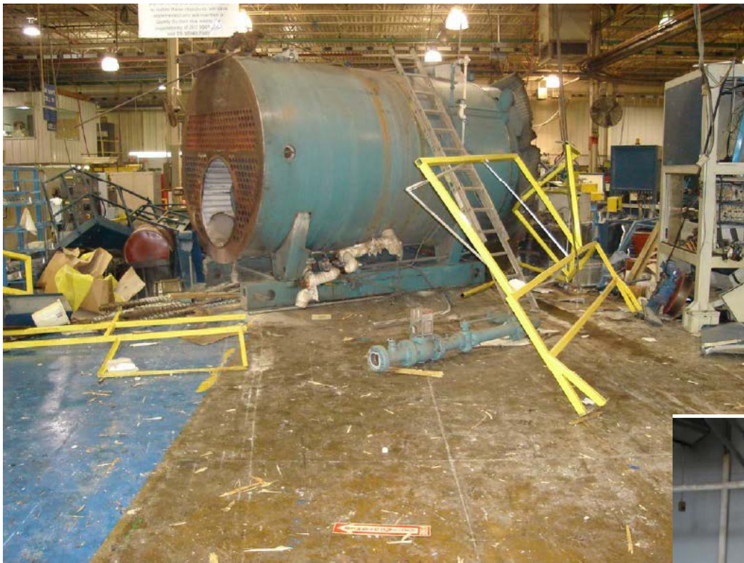
Photo #2 – Final Location of Boiler After Explosion
