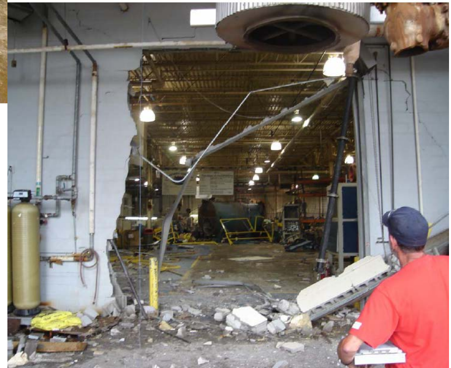
Photo #4 – Hole Created by Boiler through Roll Up Door Wall (West Wall)
