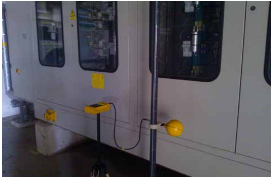
Figure 3.6 — Measurements being made near a thyristor rectifier
