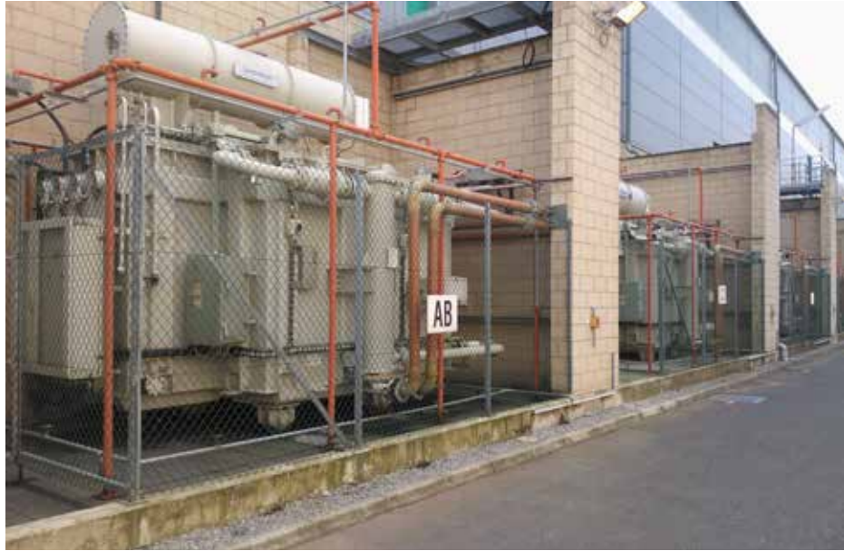
Figure 3.4 — The transformer bays
