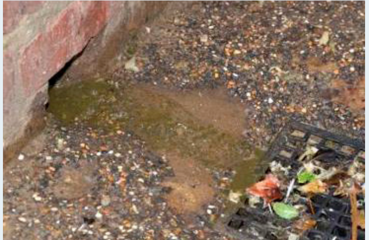
Do not allow run-off to contaminate walkways
