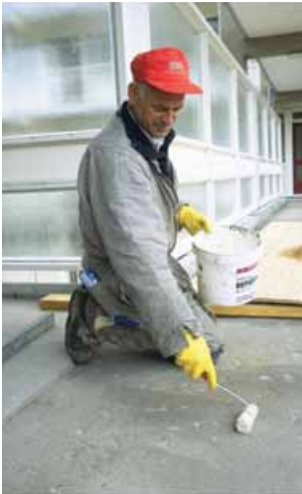
A floor coating being applied by a worker who is kneeling down and using a short-handled spreader.
