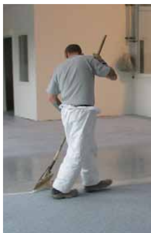
With the help of a long-handled spreader, an adequate safe working distance has been applied, reducing the likelihood of contact with the coating. It reduces the potential for back problems too.
