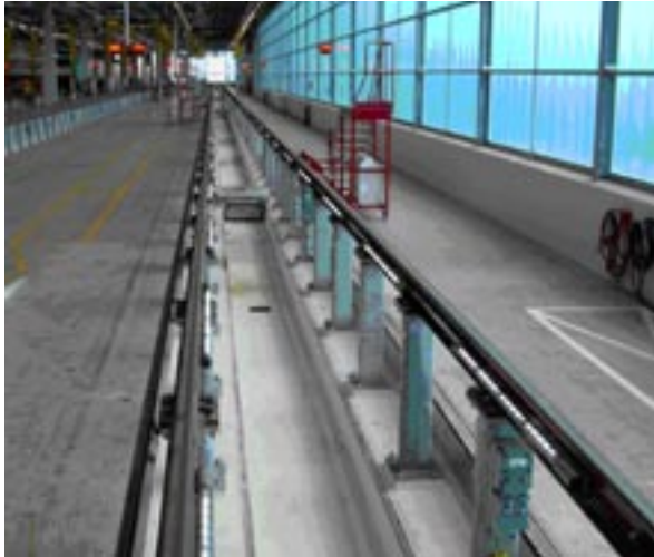
Figure 18: Rails with LEDs
