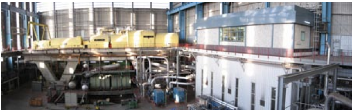
Safety and health in Langerlo
