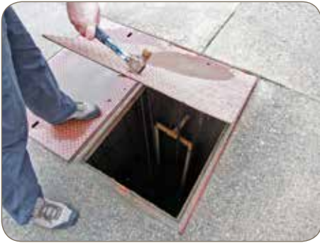
Lift station hatchway
