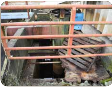
Irrigation pump station
