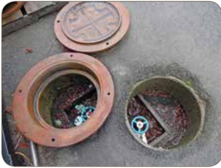
Stormwater manhole and drains
