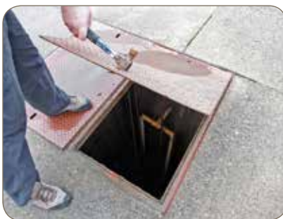
Lift station hatchway
