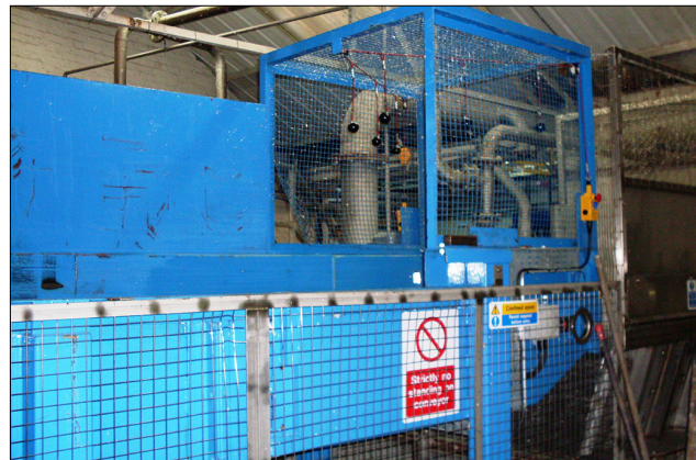
Figure 16 An example of a horizontal conveyor feeding a pulp storage tank in the stock prep area using fixed guarding and extended sides
