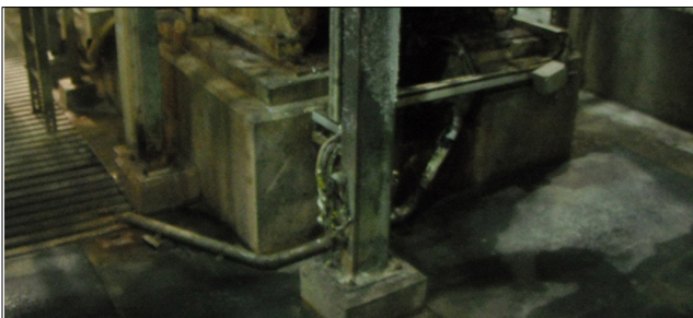
Figure 24 Contamination around the refiner being discharged into drains, cleaning will also be needed
