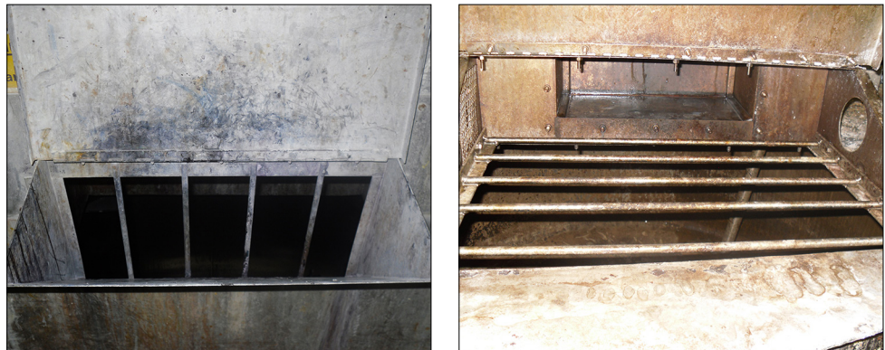
Figure 20 Example of fixed grilles on side and top openings of a pulper. Both fixed grilles have been added to prevent whole body access
