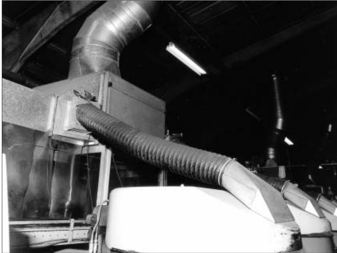
Figure 10 Tyre presses fitted with exhaust ventilation for controlling rubber fume
