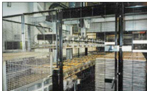
Solution: new robot installed for lidding/de-lidding tins
