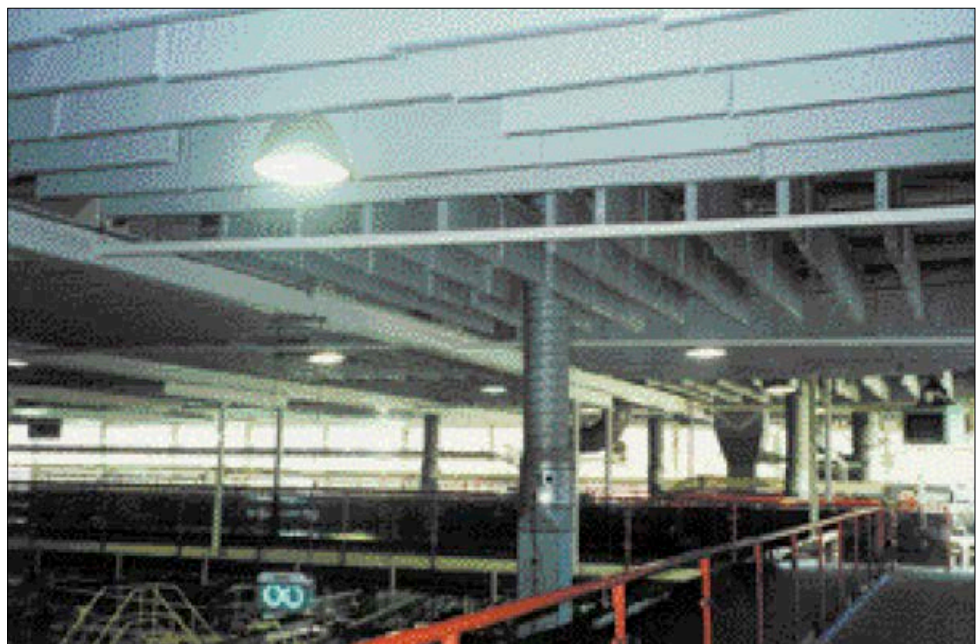
Solution: acoustic baffles fitted to ceiling
