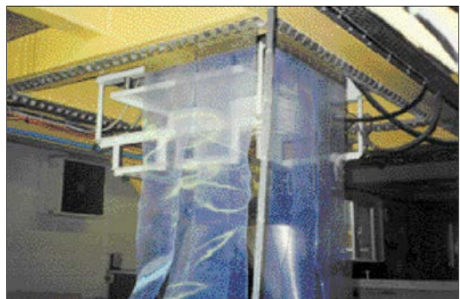
Solution: PVC curtain enclosure under construction (50% overlaps are required to be effective)
