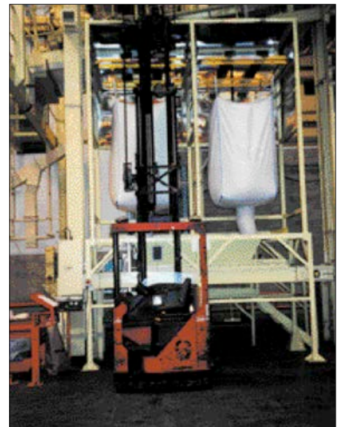
Problem: one-tonne bag of dried food suspended above original conveyor
