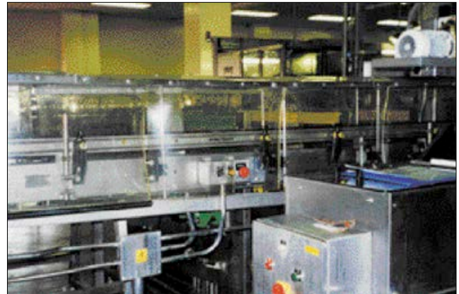
Solution: conveyor with enclosure fitted
