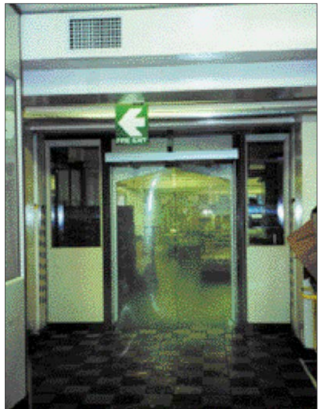
Solution: automatic, flexible PVC curtain doors installed to segregate ear protection zone from quieter area
