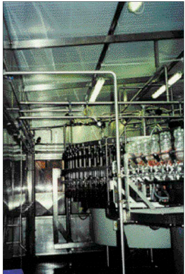
Solution: machine enclosed by large steel frame fitted with noise-absorbent ceiling and perspex sides (photo taken from within enclosure)
