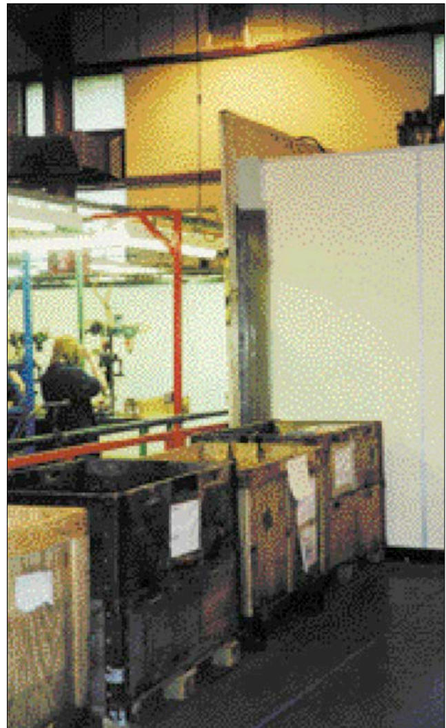
Solution: new, sound-absorbent steel sandwich wall erected between production area (left) and office (white fabrication on right)
