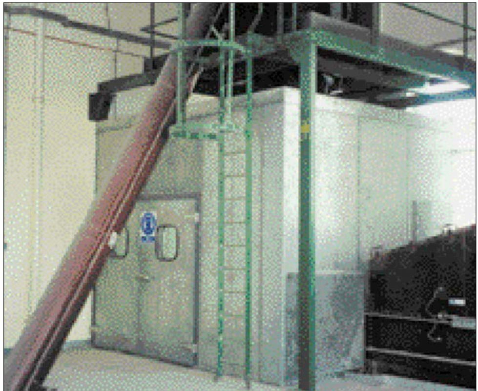
Solution: hammer mill enclosed in acoustic booth
