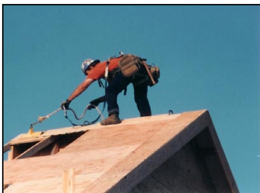
The anchor and lifeline were installed on this roof section before it was lifted into place.
