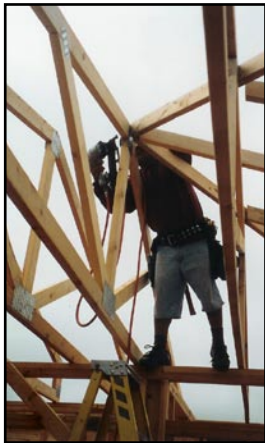
Working at the peak from the top plate of an interior wall.
