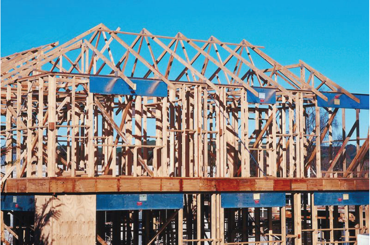
An example of an established floor . An established floor is any floor where all the exterior walls are in place.
