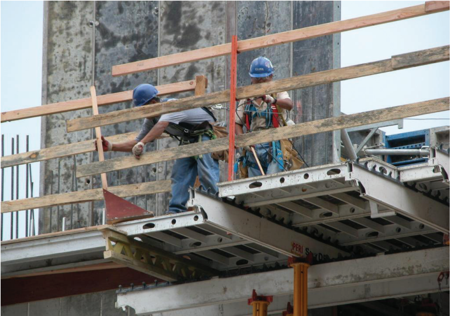
Assembling guardrails. Worker at leading edge tied off to a retractable lanyard.
