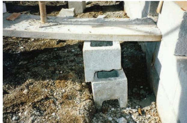
Never use bricks or blocks to level a scaffold.
