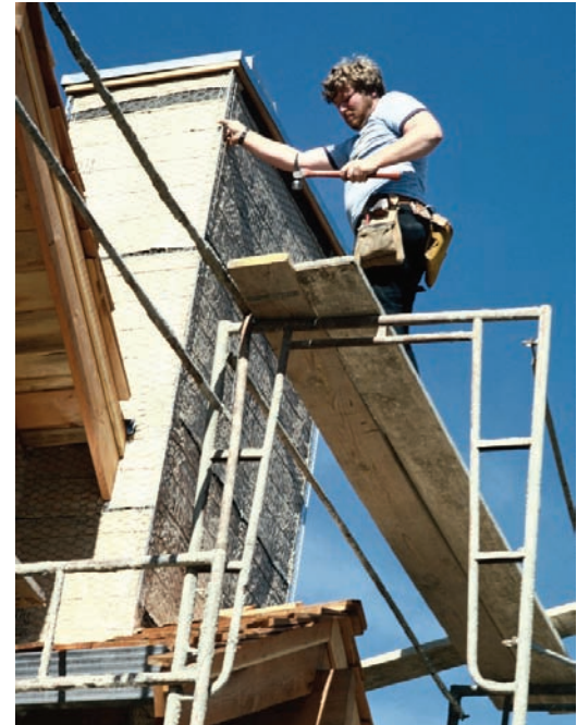
Fall Hazard! No guardrails. This scaffold has no guardrails and is not fully planked. If you work on a supported scaffold more than 10 feet above a lower level, you must be protected from falling.
