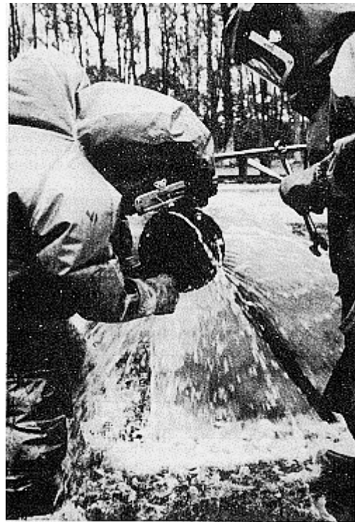
The training program should involve field drills that simulate emergency situations. Here workers wearing Level A personal protective equipment repair a leaking pipe as part of a training exercise.
