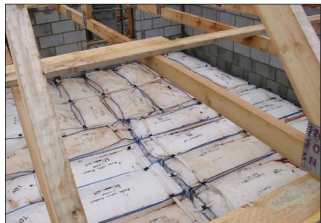
Figure 15(c) Bean bags being used as a fall mitigation measure during roofwork (Image courtesy of Forest Safety Products Ltd)
