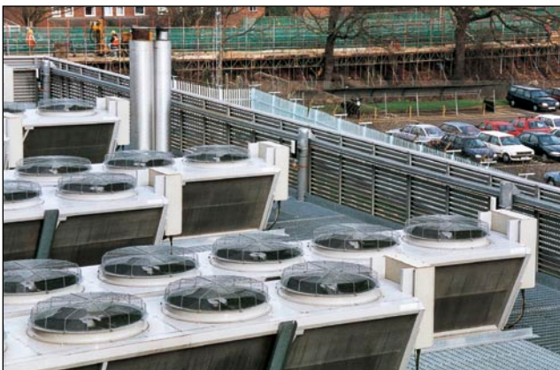
Figure 44 Parapet edge protection included as an integral design feature
