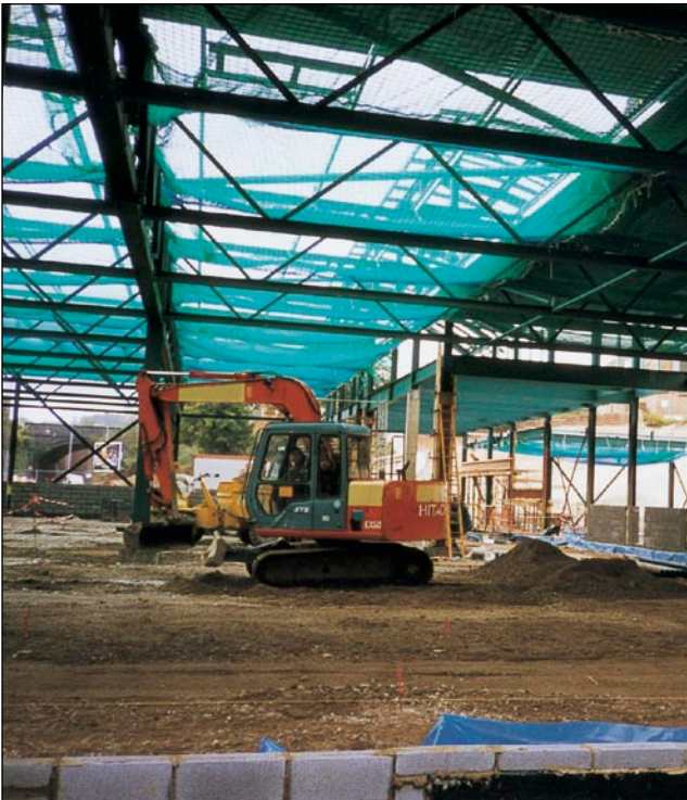
Figure 8 Debris netting used in addition to safety netting may enable work to be carried out safely below roof workers
