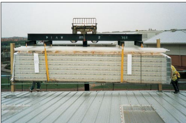
Figure 34 Delivering sheets to roof level onto the completed load-bearing section and behind the leading edge. (Note that the roof lights include mesh protection and are non-fragile)
