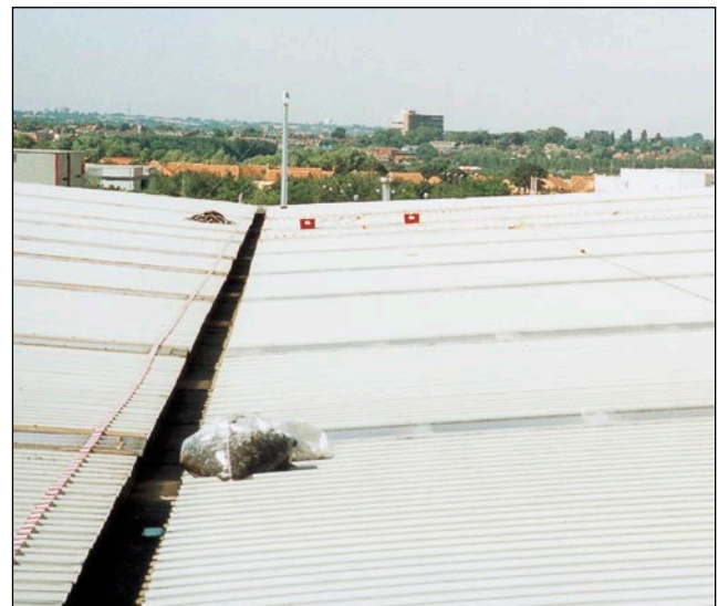
Figure 30 In some light conditions, it is difficult to distinguish the roof lights from the metal sheets on this type of roof. The valley gutter is very narrow and roof lights extend down to gutter level. Both of these features increase the risk during cleaning, maintenance or refurbishment
