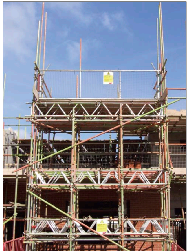
Figure 35 Loading bays should be designed for the actual weight of the materials to be placed on them and include an additional allowance for impact loads from mechanical handling (eg cranes or forklifts). A notice should clearly display the safe working load
