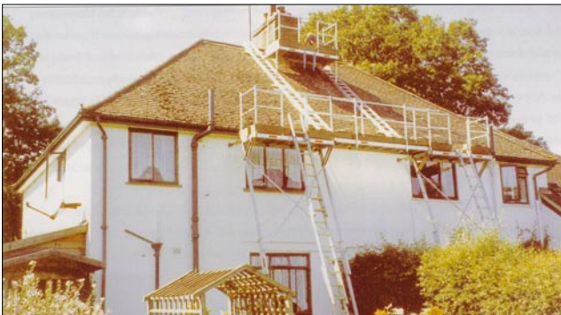
Figure 3 Proprietary access system for roof work
