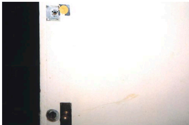
Figure 48c Painted asbestos insulating board facing to a fire door with some damage around the door furniture
