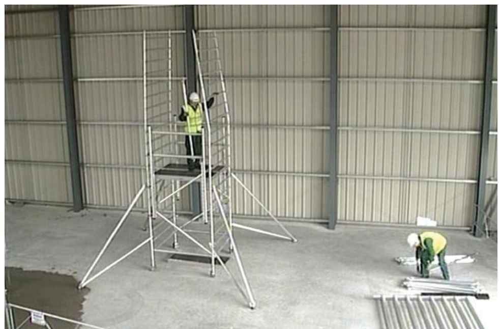
Figure 11 Advanced guard rails
