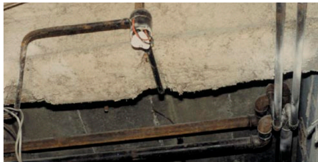
Figure 48b Poorly tamped sprayed chrysotile fireproofing on a structural steel beam holding up a concrete floor, showing some overspray onto the concrete and damage by electrical work
