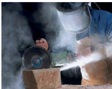
Photograph 2 Disc cutting. End of disc cutting through a stone block. Jets of dust-laden air are very fast moving and difficult to control (see also Figure 11)
