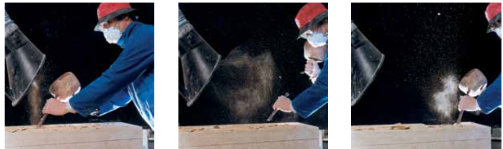
Photograph 6 Hand chiselling and captor hood exhaust ventilation. Sequence of three photographs shows stonemason working within the hood capture zone, partially within it and well outside it. Dust control is only effective when work takes place within capture zone (see Figure 14).
