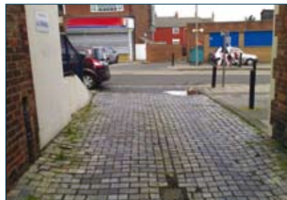
Figure 6 Narrow and uneven driveway for delivery vehicles
