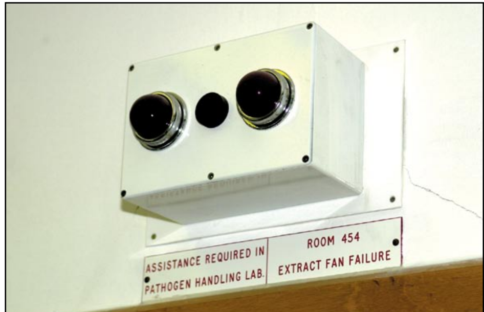
Figure 2 Alarm to indicate fan failure
