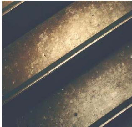
Picture 7: Anti-skid strips on the stairs
