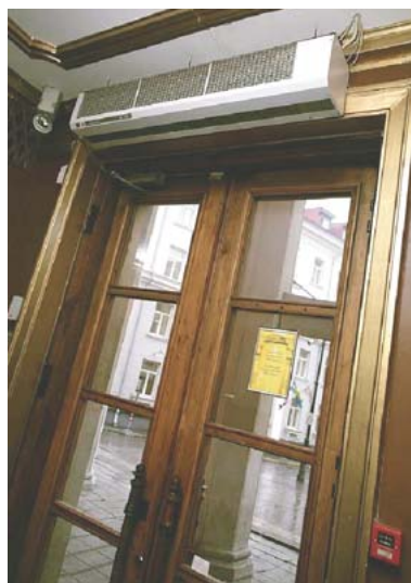
Picture 6: A blast heater at the entrance
